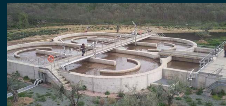
Galindo WWTP in Bilbao
